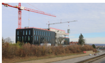
The facade modules are prefabricated, making it easy for site workers to incorporate them into the building
